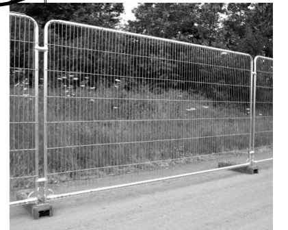
FENCE TO BE ERECTED THROUGHOUT WORKS TO PROTECT TREES
